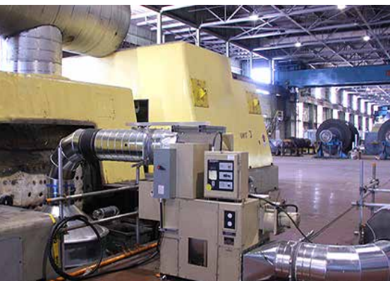
A dehumidified air system at Lambton GS minimizes corrosion of the turbine shaft and blades.
