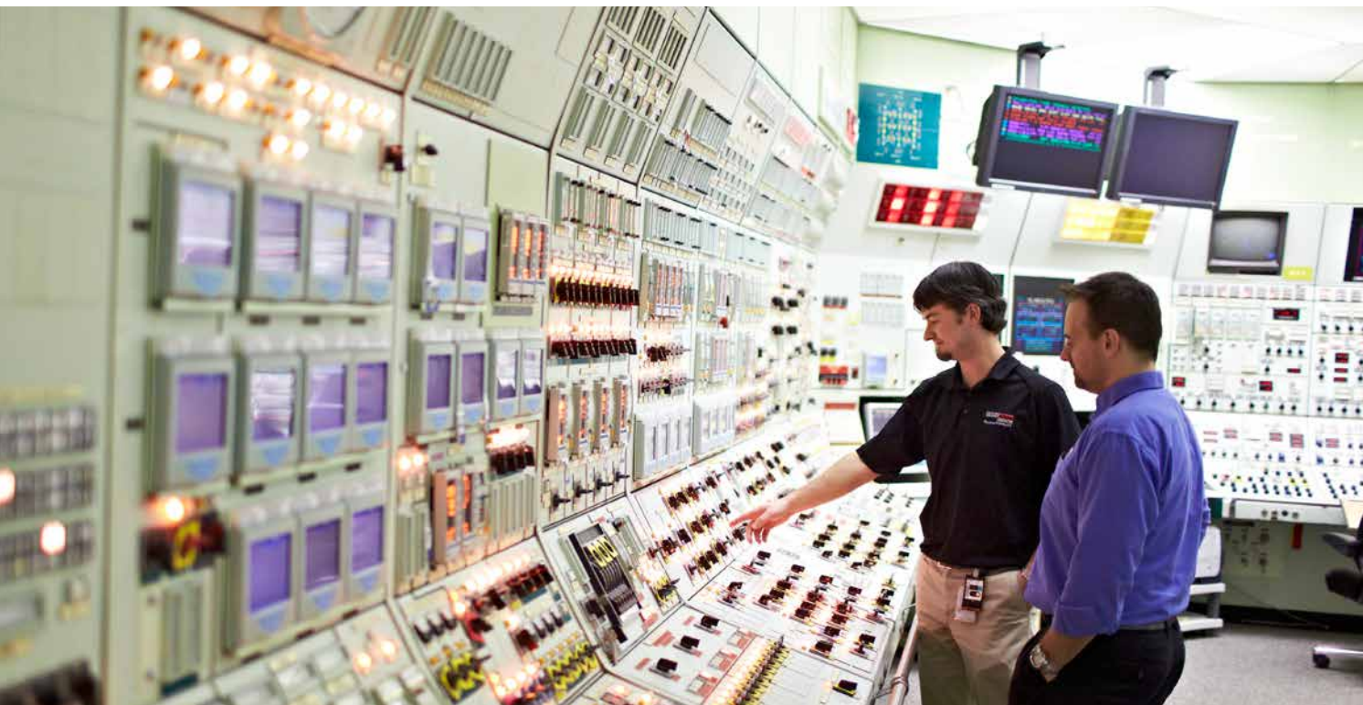
Control Room at Pickering Nuclear
