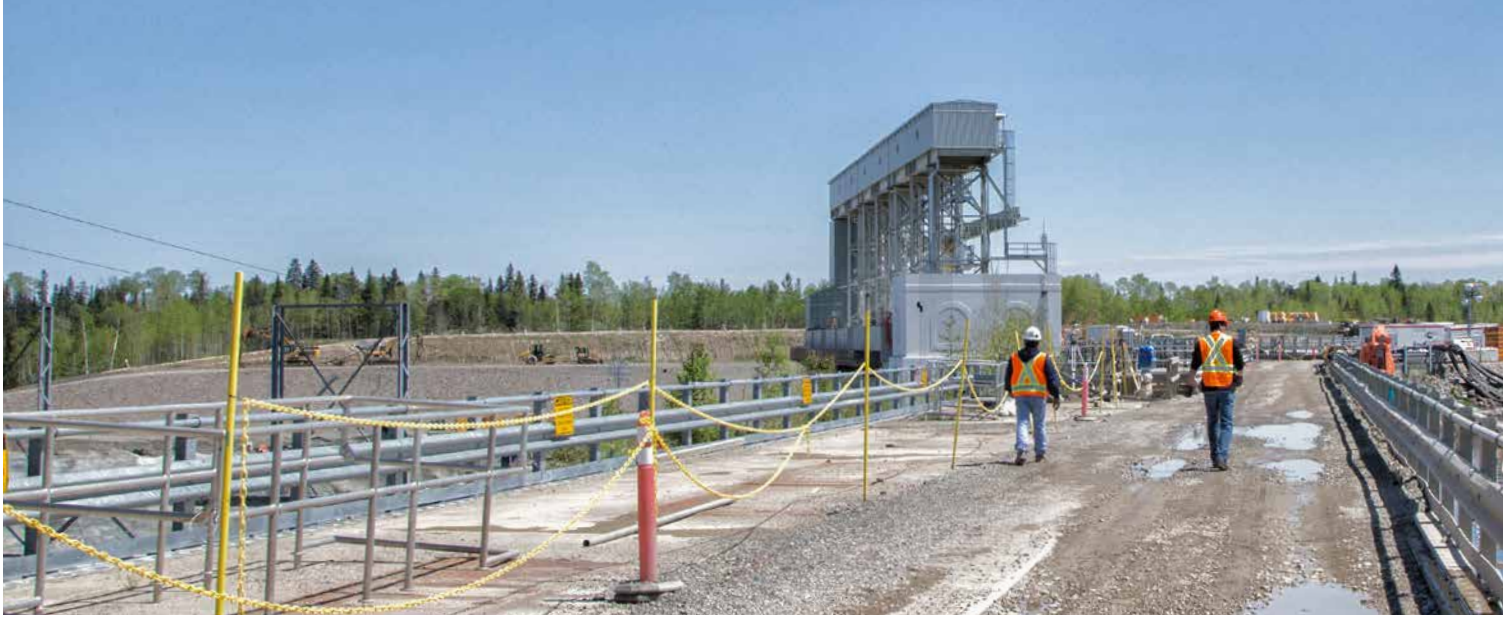
Construction of a new station at Smoky Falls, also known by its Cree name, Kâpâškiletehk, replaces the existing Smoky Falls station.
